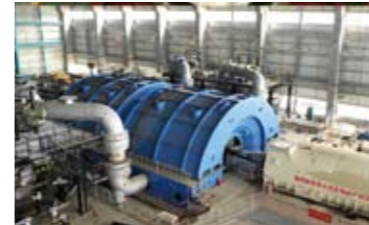
汽轮发电机组 Turbine-generator Unit
